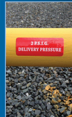
Sample of piping label used to identify elevated delivery pressure piping.
